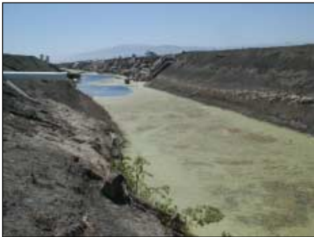
Figure 6-5. Location: Reach 1 Section 3, showing incised channel, bank erosion, and agricultural drainage pipe (Photo: Joel Casagrande)
