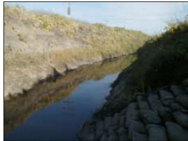
Figure 6-6. Location: Reach 1 Section 4, showing deeply incised channel, lack of riparian vegetation, and rip-rap with sand bags (Photo: Julie Hager)
