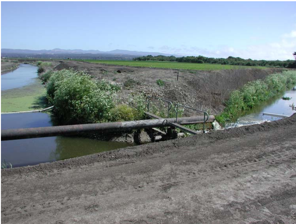
Figure 2.5. Site #4-Blanco Drain looking upstream (left) from pump-out station and downstream (right) to the Salinas River. (Photo: Don Kozlowski, June 2002)
